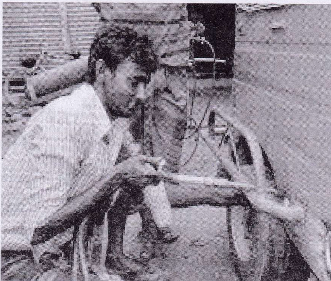
Fig.1: Worker is doing gas welding without safety
