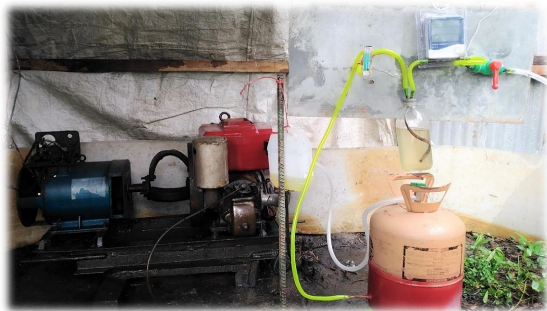
Fig.4.12: Dual fuel Setup Project picture 2
